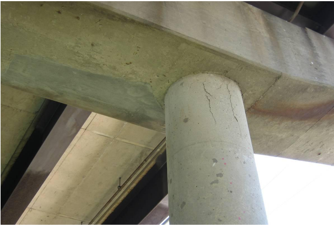
Photo No. 48 Pier 8, delaminations at top of west column, looking SW
