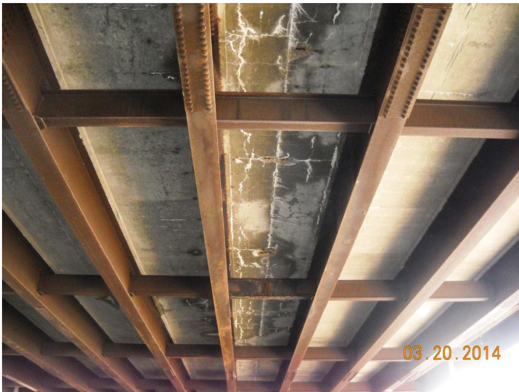
Photo No. 32 Bottom of deck and beams, span-16 – center bays, looking south
