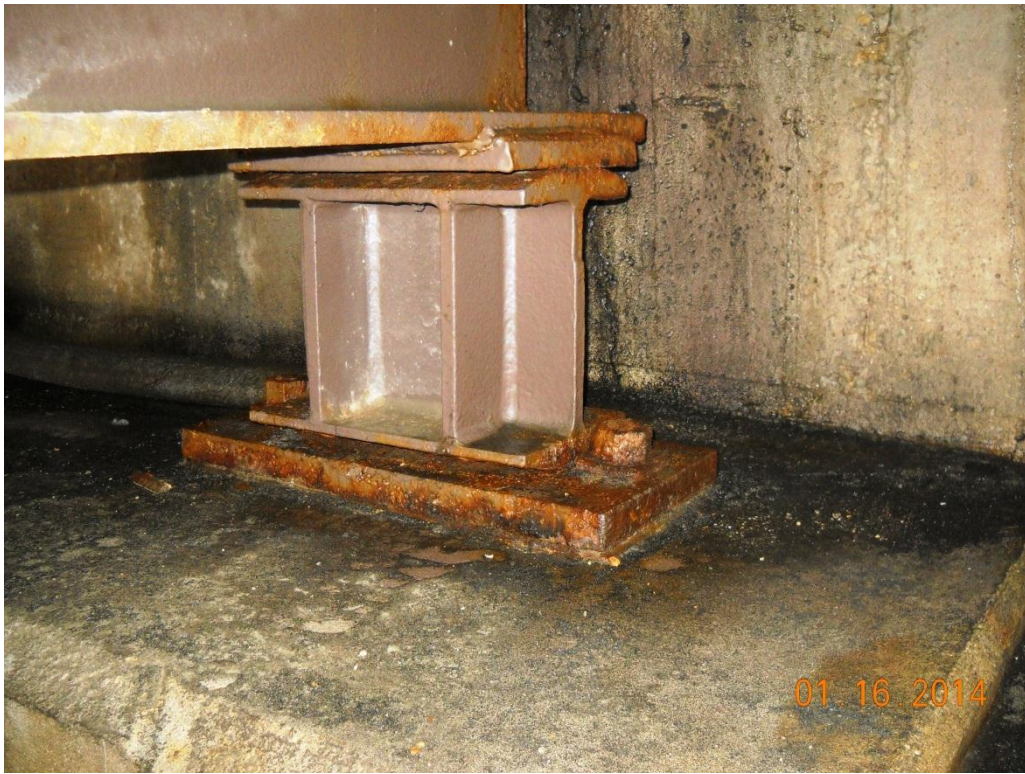
Photo No. 36 Expansion bearing at north abutment – typical condition
