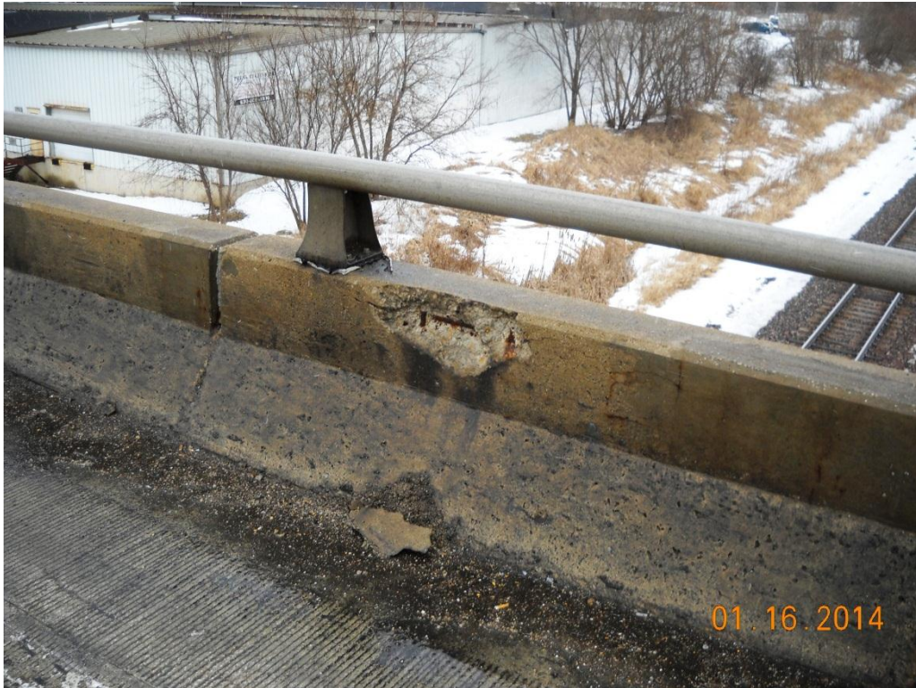
Photo No. 17 Spalled concrete on parapet - common
