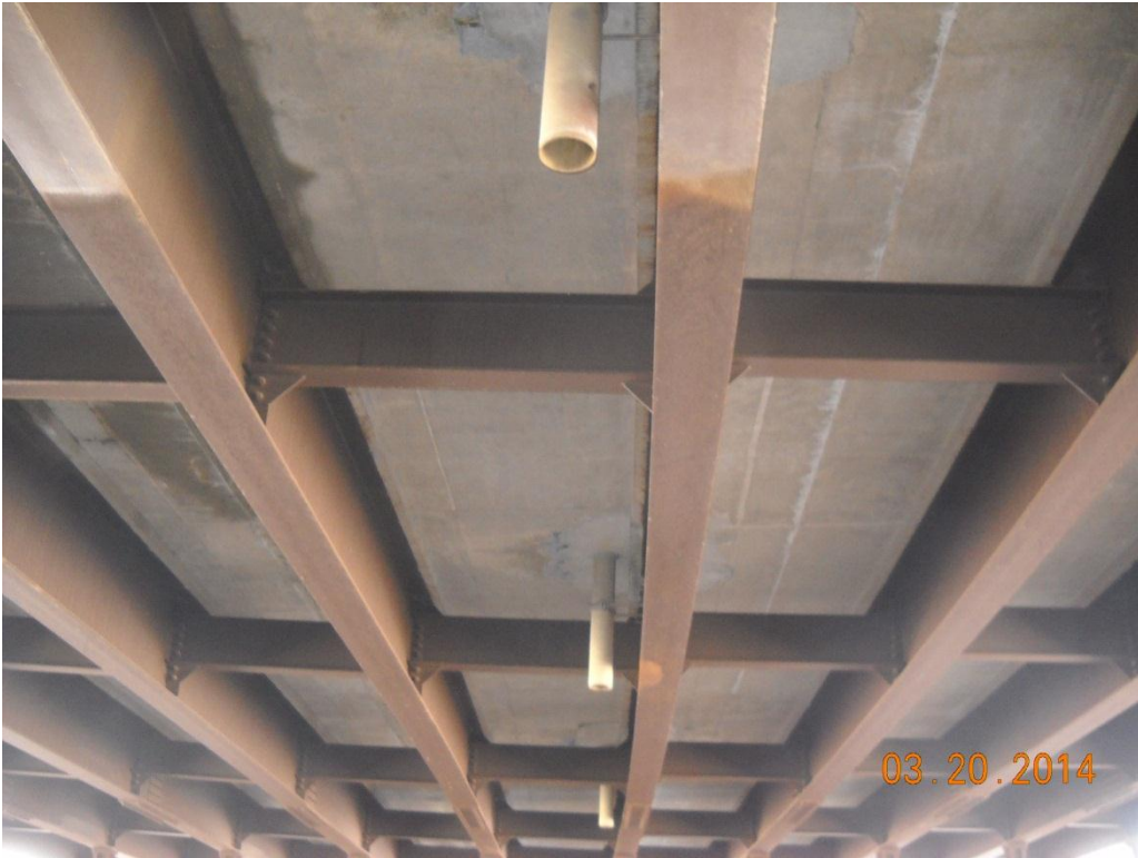
Photo No. 29 Bottom of deck and beams, span-4 – center bays, looking south
