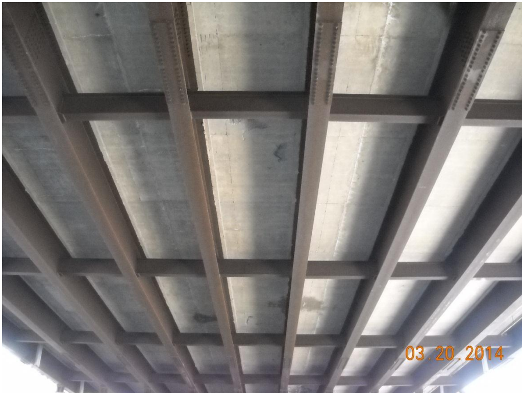
Photo No. 31 Bottom of deck and beams, span-15 – center bays, looking south
