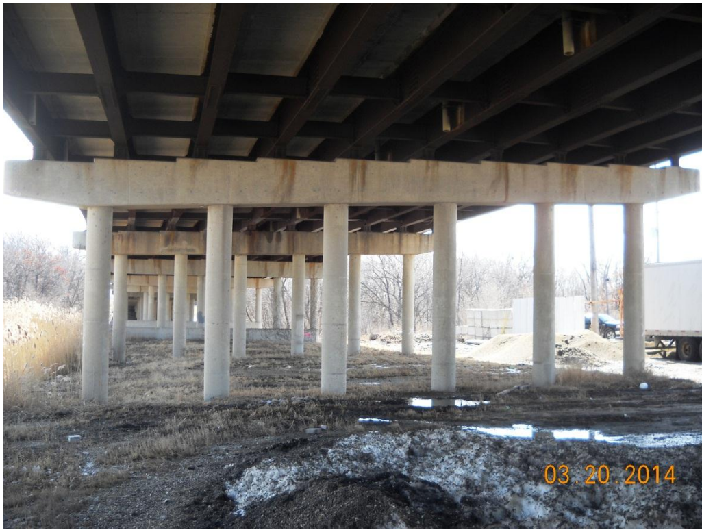
Photo No. 46 Pier 7, looking south (typical pier condition without transverse deck joint)
