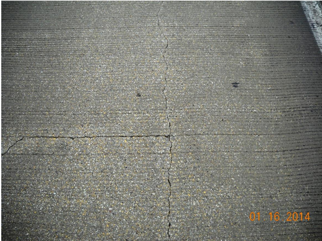
Photo No. 19 Top of deck, span 5 SB – intersecting open cracks in overlay (common)
