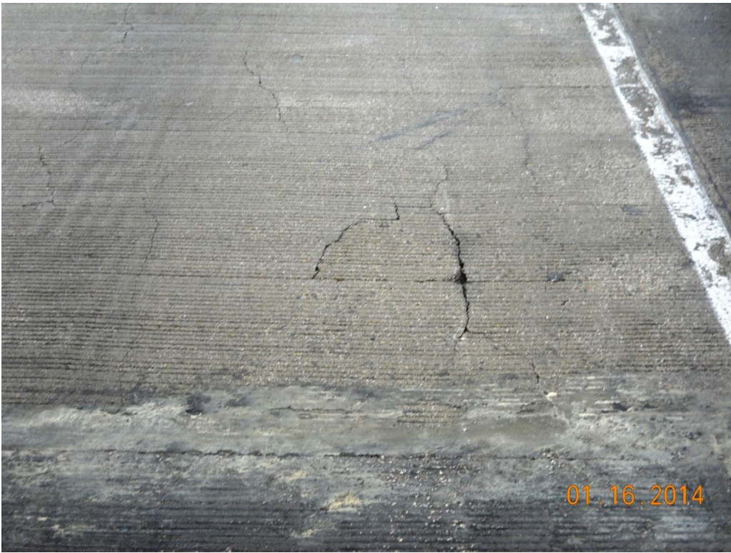
Photo No. 26 Top of deck, span-3 – intersecting open cracks in overlay
