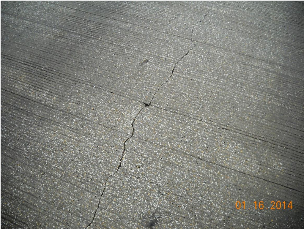
Photo No. 21 Top of deck, span 9 SB – open cracks in overlay (common)
