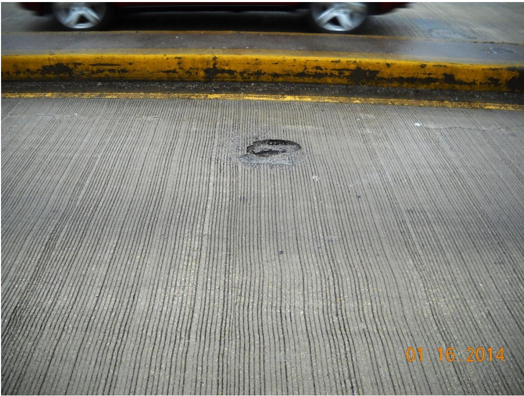
Photo No. 22 Top of deck, span 16 SB - spall
