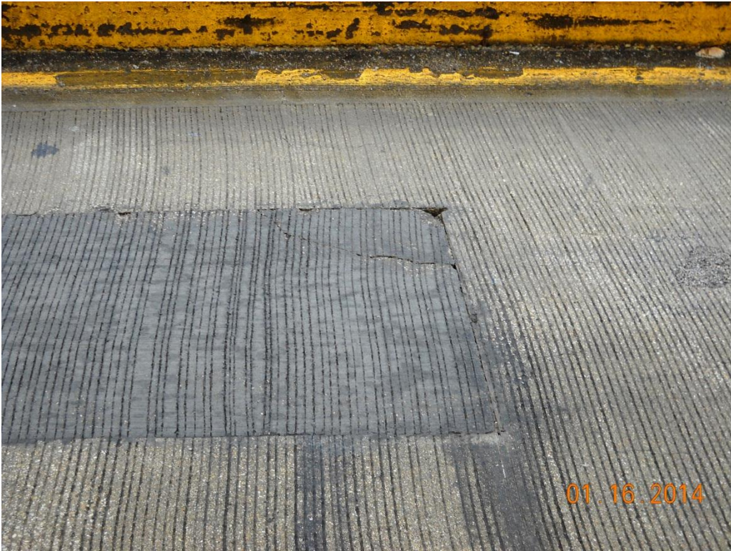
Photo No. 25 Top of deck, span-7 NB, damaged concrete patch
