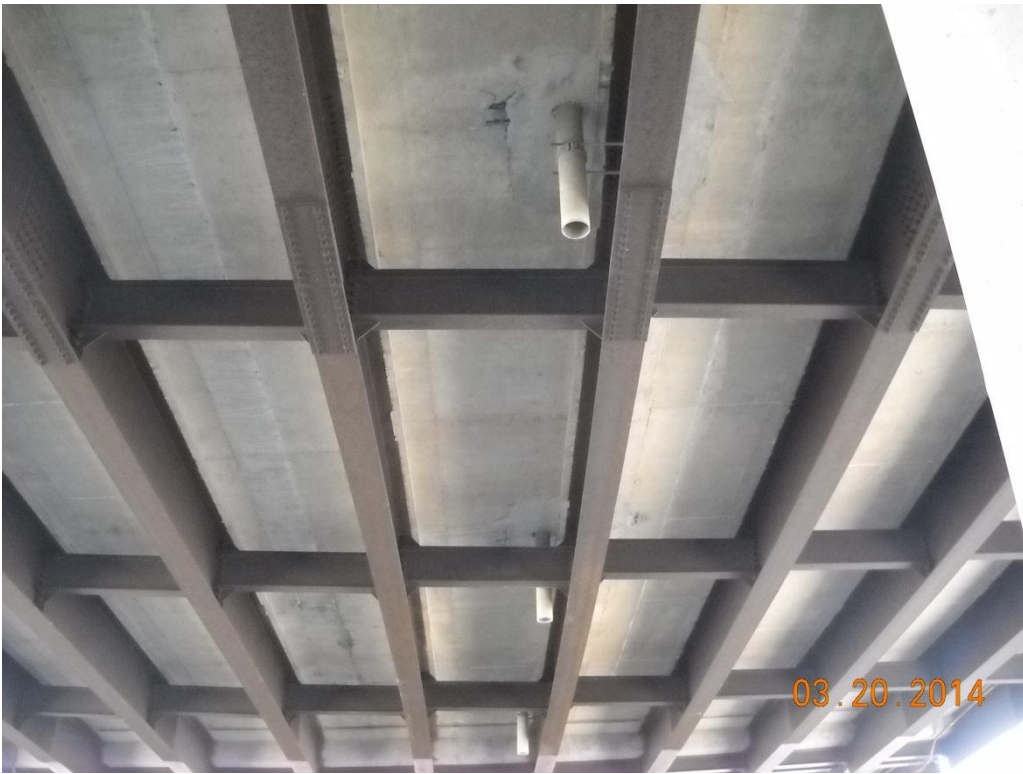
Photo No. 30 Bottom of deck and beams, span-8 – center bays, looking south
