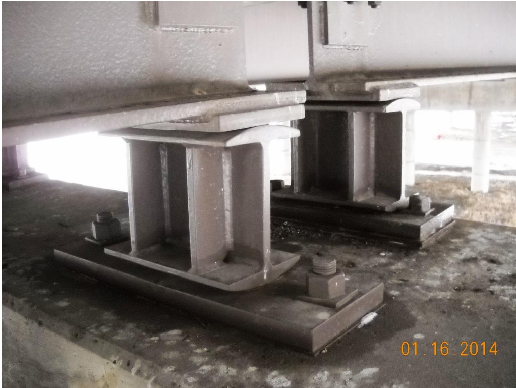
Photo No. 37 Expansion bearings at Pier-3, typical condition beneath interior transverse joints
