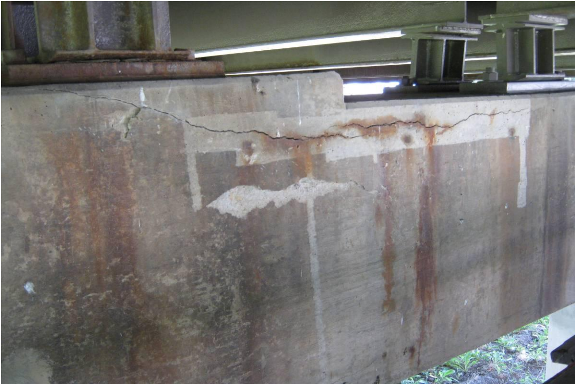
Photo No. 45 Pier 3, looking SW, cracking and delaminations common in cap
