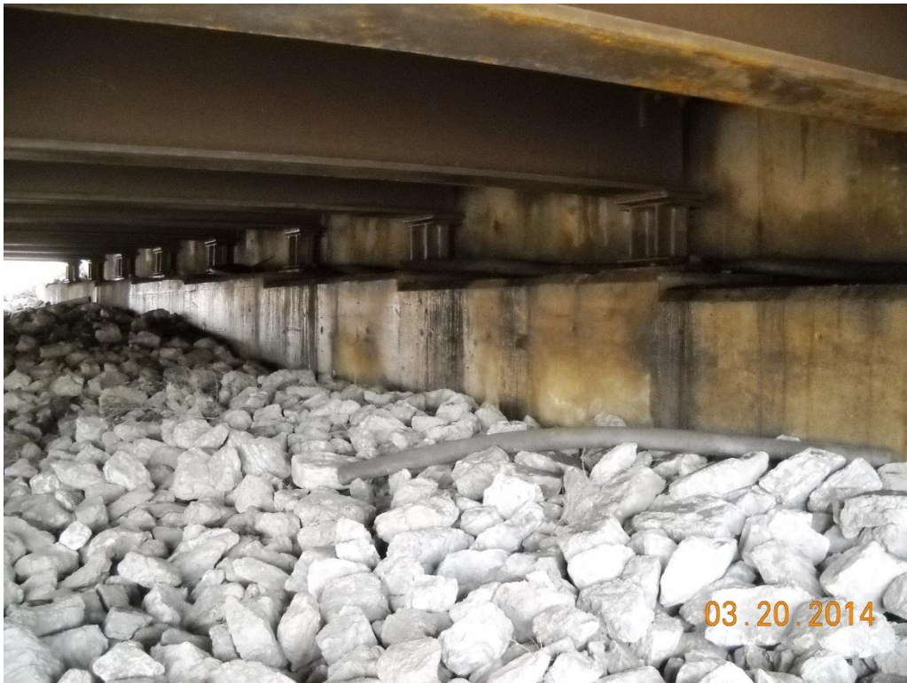
Photo No. 41 Abutment cap – typical condition
