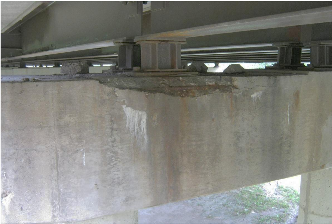
Photo No. 50 Pier 13, east end looking south, spalling and delaminations common in cap
