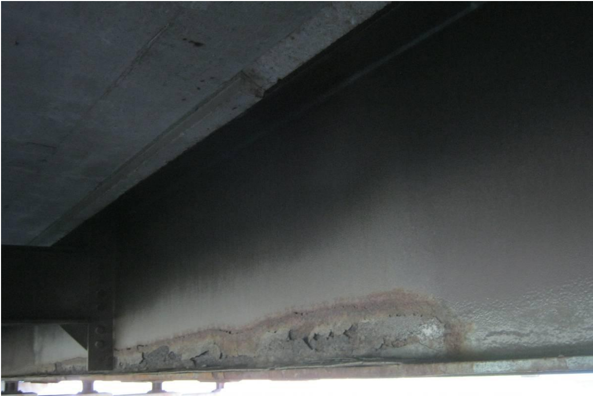
Photo No. 39 Corrosion on web and bottom flange on Beam-6 from west side near Pier 3
