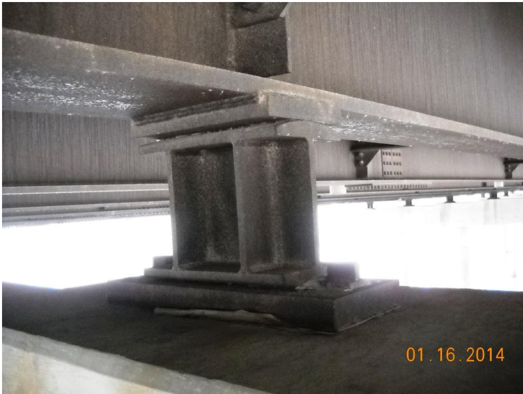
Photo No. 38 Expansion bearing at Pier-5, typical condition beneath continuous deck locations
