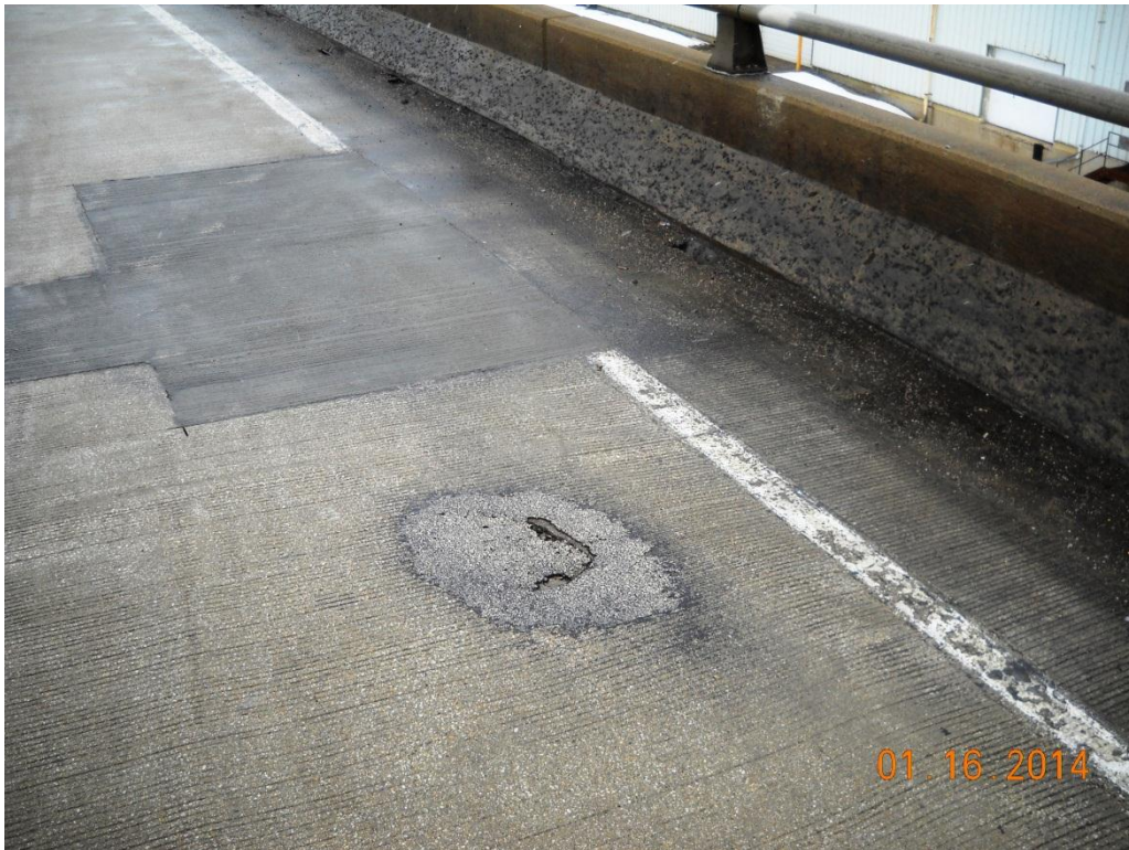
Photo No. 24 Top of deck, span-7 NB, oil and chip patch
