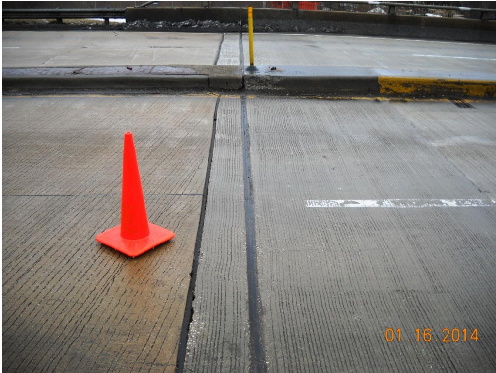
Photo No. 9 North abutment transverse joint, seal is leaking
