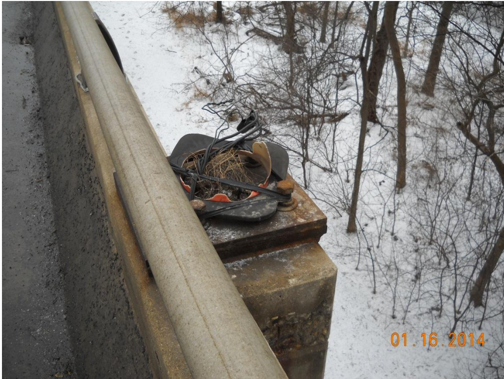
Photo No. 27 Missing light pole, span-14, west side
