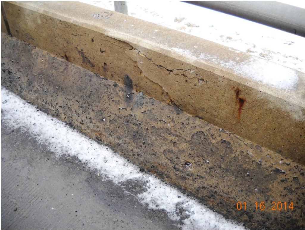
Photo No. 16 Delaminated concrete on parapet - common
