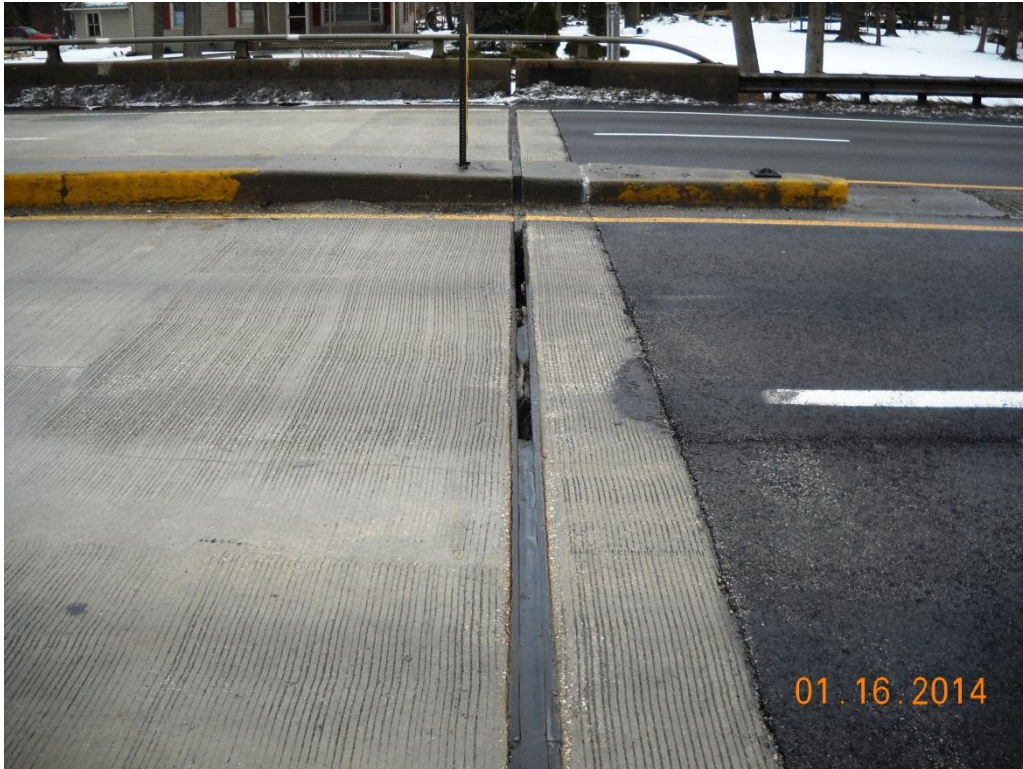
Photo No. 13 South abutment transverse joint, seal has failed
